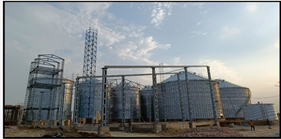
12,500 MT x 3 WHEAT Silos, 3000 MT x 4 RICE Silos Grain Terminal
